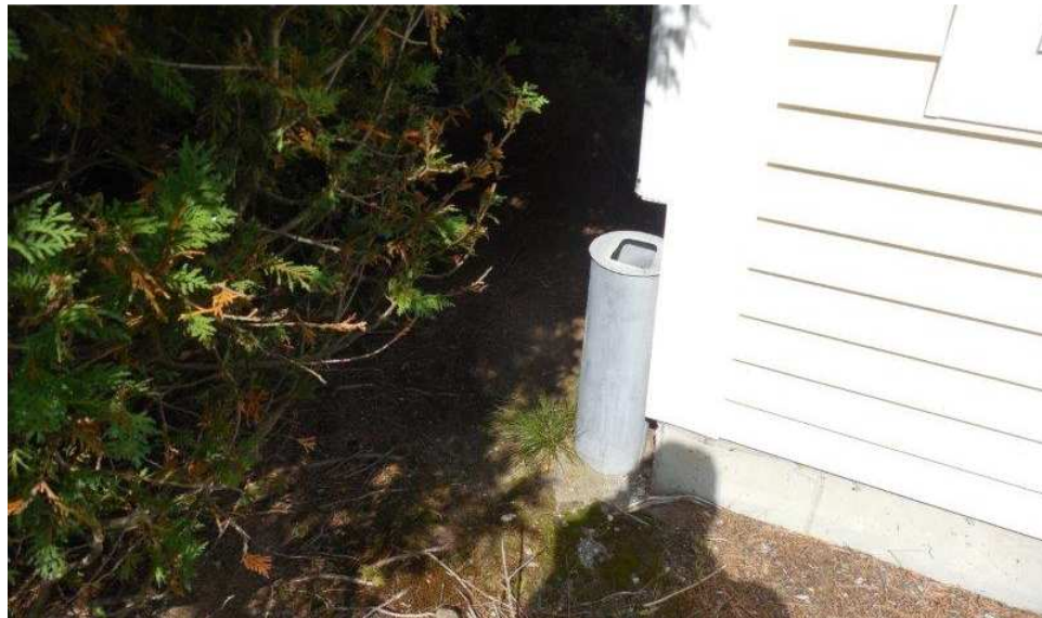
disconnected drain riser
