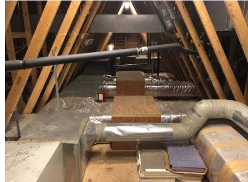
ductwork in attic
