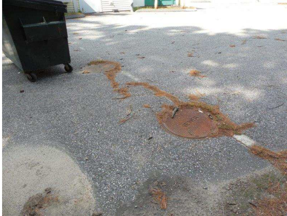
manhole covers near dumpster pad
