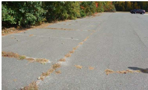
overgrowth at parking lot
