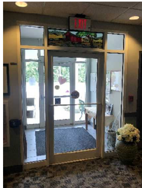
power door operator at front entry
