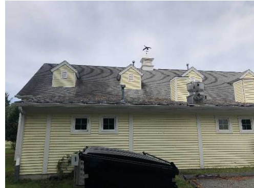
stained roof shingles
