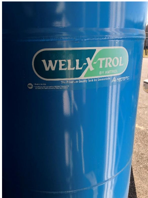
PL-2 Domestic Water Well Pump Storage Tank
