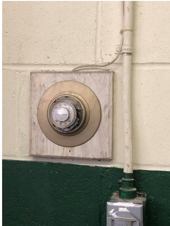
M-4 Thermostat Controls
