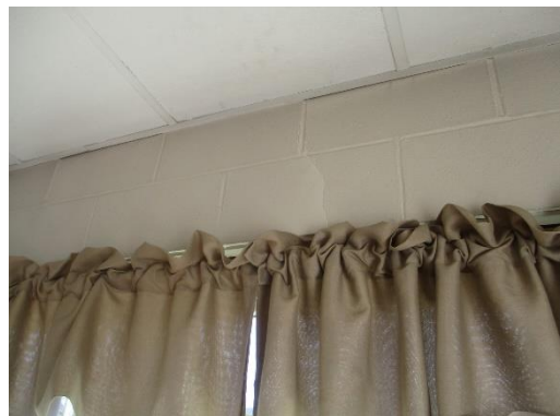
12 – Cracks in Radio Room from water damage
