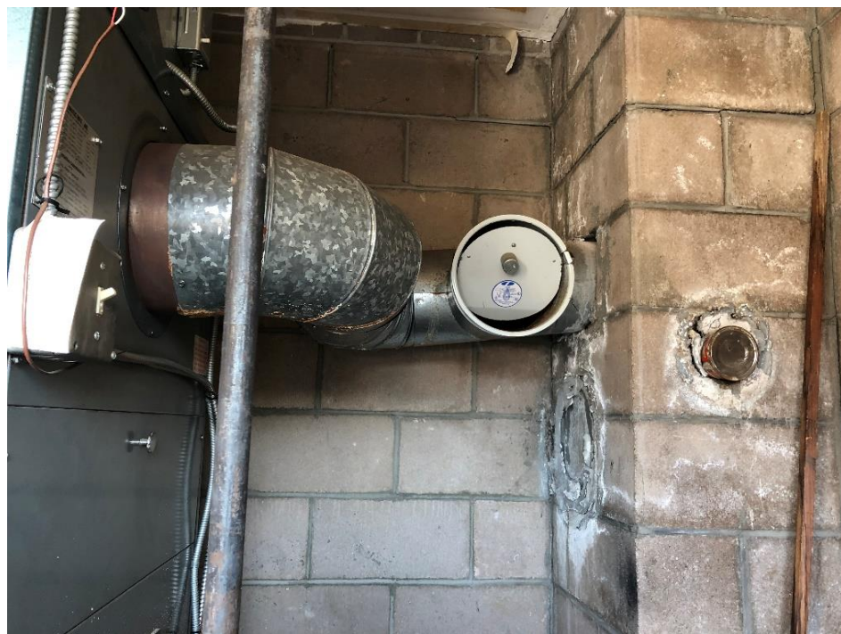
M-6 Furnace Breeching and Chimney
