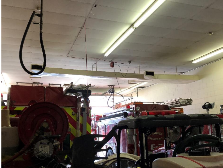
M-5 Heating Duct from Furnace to Apparatus Room
