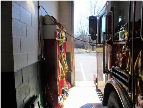
07 – Lack of electric drop reels creates hazard
