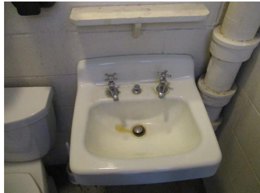
10 – Restrooms old and beyond repair
