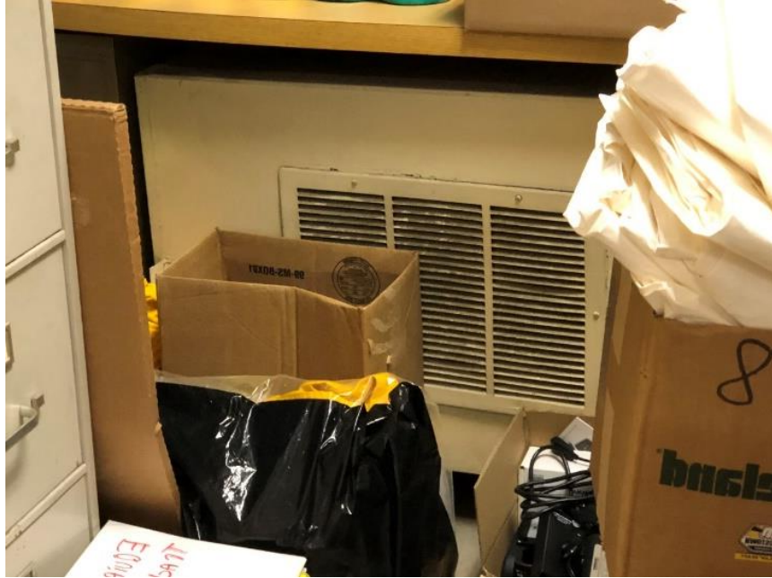
M-9 Return Grill from Apparatus Room
