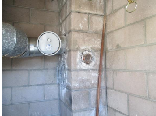
04 – Efflorescence all over chimney flue
