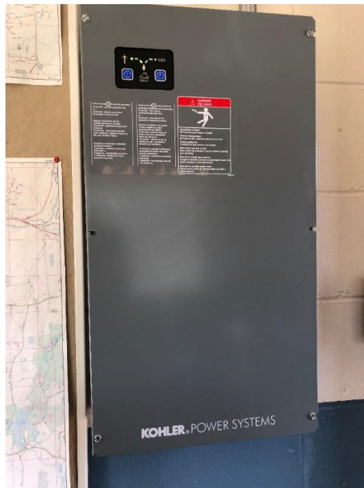
EL-13 Gen. Transfer Switch
