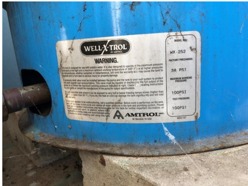
PL-1 Domestic Water Well Pump Storage Tank
