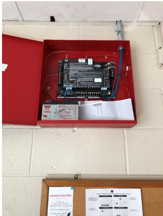
FA-1 Bosch Fire Alarm Panel
