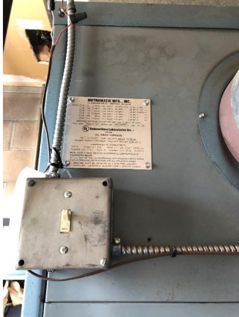
M-1 Heating Furnace Shutoff
