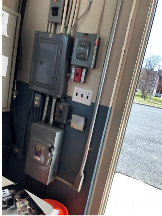
EL-3 Main Service Panels/Switches
