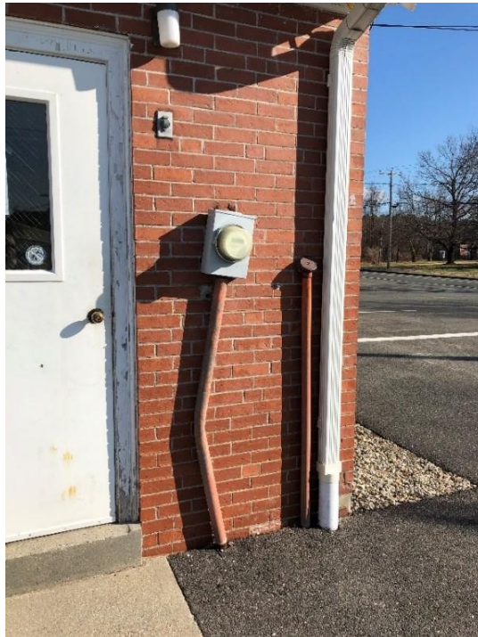
EL-2 Damaged Service Meter
