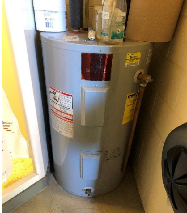
PL-4 Hot Water Heater
