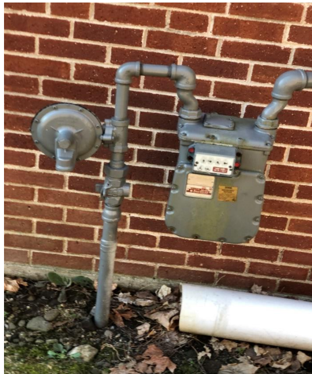
PL-9 Utility Gas Meter
