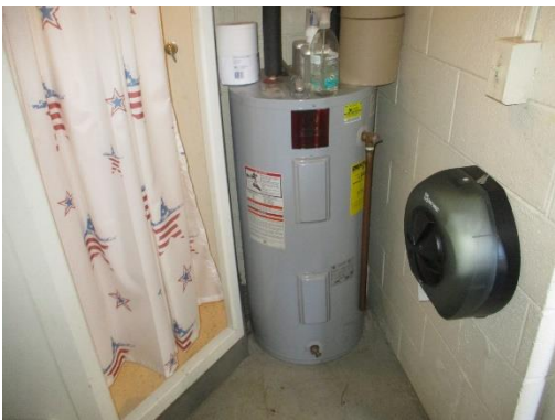
09 – Water heater located in Bay Bathroom
