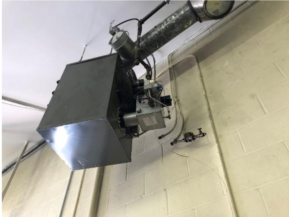
M-7 Unit Heater Exhaust Duct
