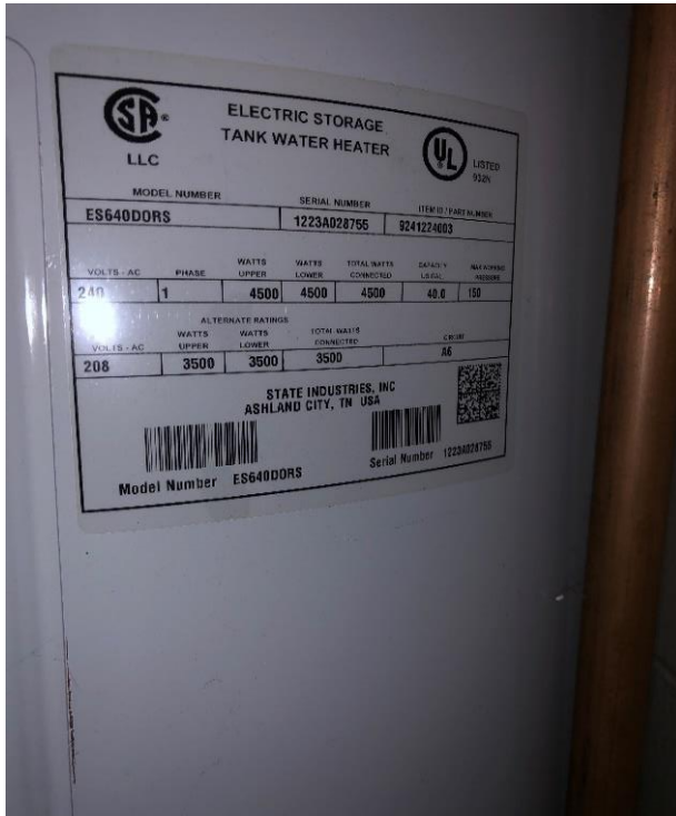
PL-5 Domestic Hot Water Heater Nameplate
