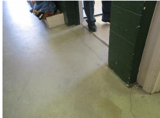
02 – Various Bay and floor slab cracks
